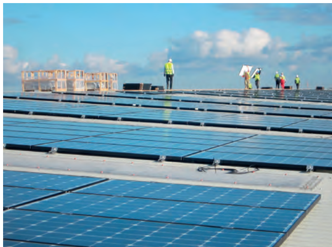
Big three: Hitachi Rail Europe's 1MW PV array in County Durham has been financed under an innovative funding framework in conjunction with Photon Energy and Macquarie Lending
