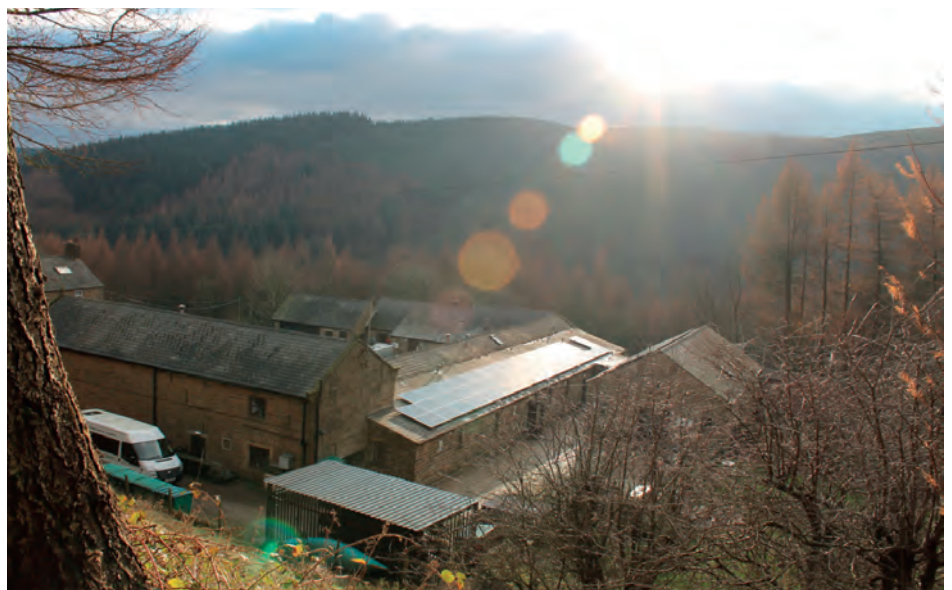
Tough task: Nottinghamshire County Council and Evo Energy overcame a 7kWp export limit on its 32kWp rooftop array at Hagg Farm with an innovative EPC system
