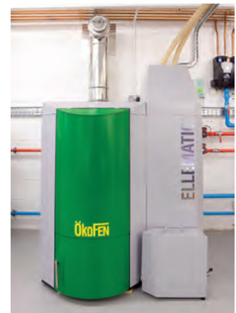
Loan star: Perthshire hotel owners Neil and Catriona Menzies have secured long term cost savings by switching to ÖkoFEN Pellematic wood pellet boilers, facilitated by an Energy Saving Trust interest free loan
