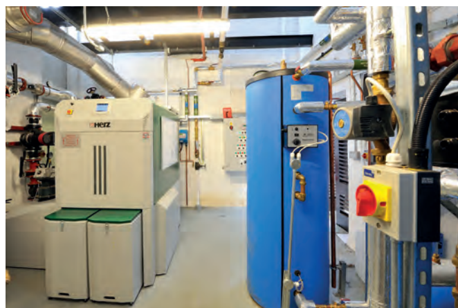
Community spirit: The Hamworthy Herz Firematic biomass boiler (left) and Powerstock Calorifier (right) along with other equipment provide the heating and hot water for Fairstead Community School
