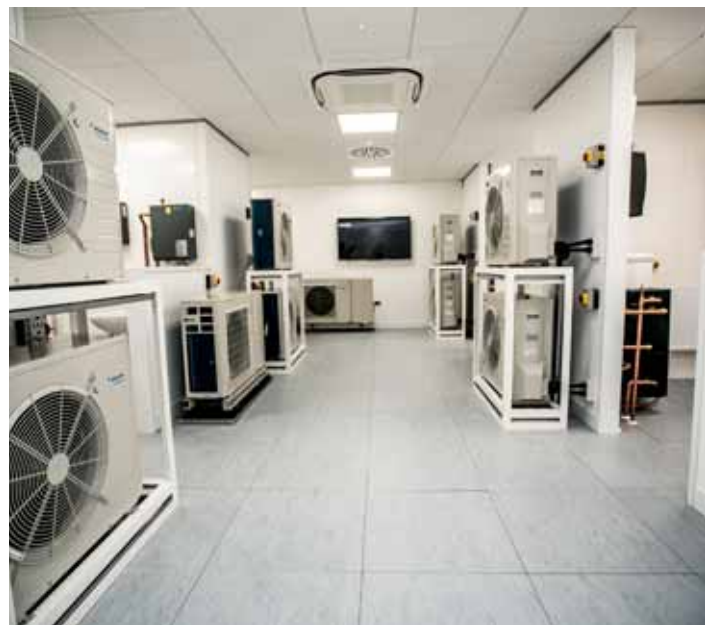
Well spent: Daikin UK has responded to the predicted skills shortage in the HVAC industry by investing £1.1m in its new national training centre in Woking
