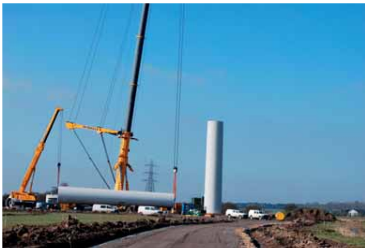
Flood mitigation: Sykes Pumps were tasked with protecting the Bradwell-on-Sea wind farm during its vulnerable construction phase, and thereafter
