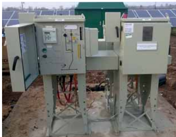
Fast movers: Lucy Electric needed just four weeks to install switchgear at two 3,000kVa solar farms, developed by Green Switch Solutions
