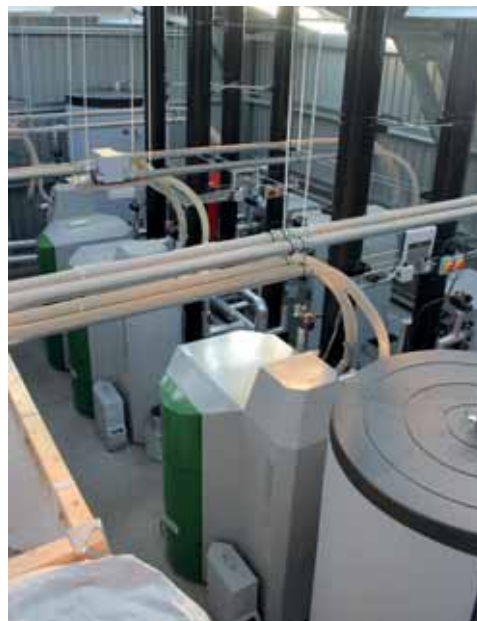
New order: The Stones Hotel, Swindon, has swapped LPG for a more sustainable wood pellet system
