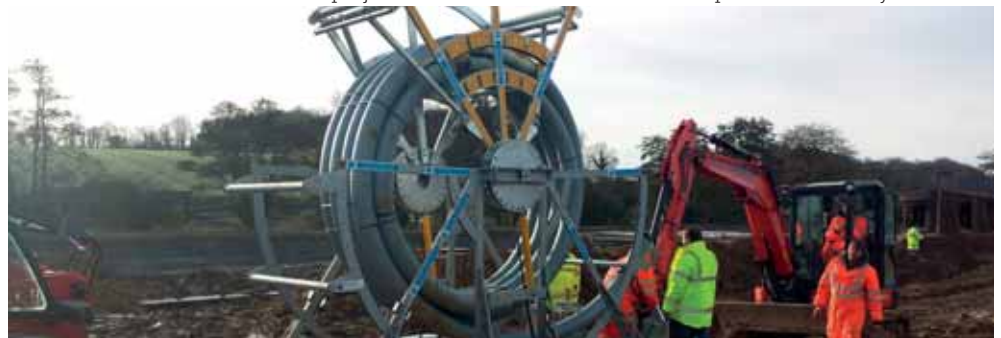
Pipe dreams: Treco opted for REHAU RAUTHERMEX pipework due to low heat losses on one of the UK's largest district heating projects, in rural Oxfordshire
