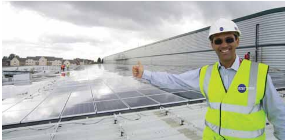
Aiming high: Azur Solar md, Robert Markus Feldmann, intends to double the Slough-based company’s annual revenues to £20m
