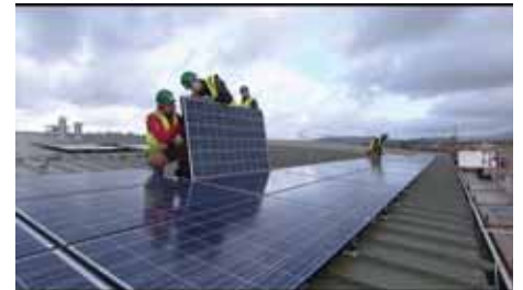
Hot news: Sundog Energy says this PV installation is the largest in Cumbria
