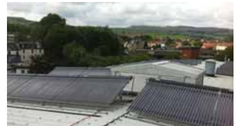
Making music: Radio City's new solar thermal vacuum tubes from Kingspan Renewables have proved successful
