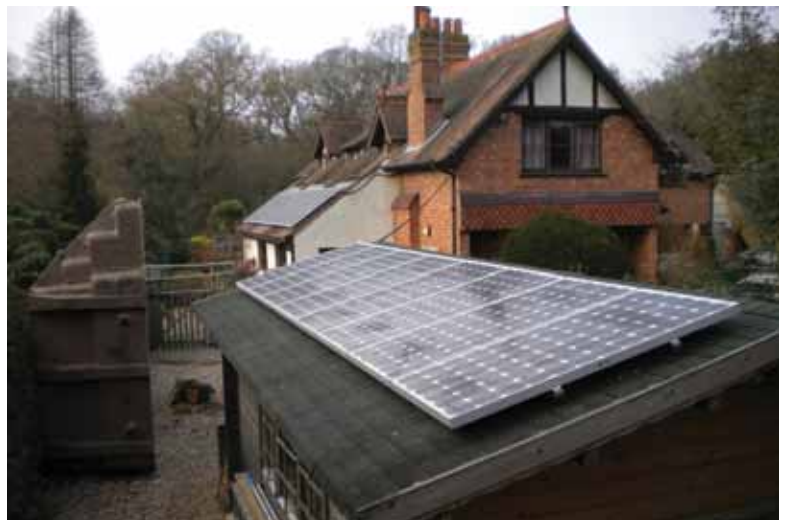
Top it off: An installation using SolarEdge power optimizers
