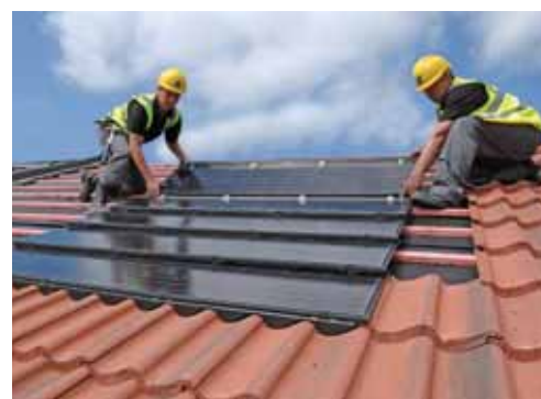
Leading by example: Brechin-based roofing specialists Forster has installed PV on the roof of its head office
