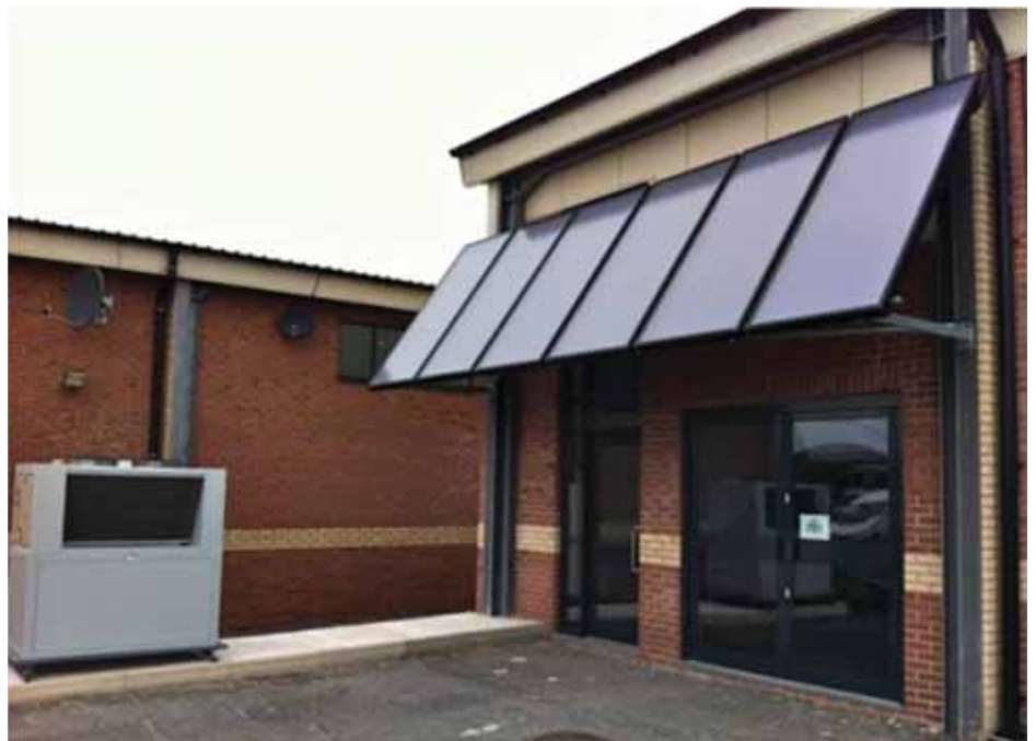
Hot stuff: A 20kW unit. This is a demonstration site with the unit connected to a Ratiotherm cylinder providing energy for a district heating scheme
