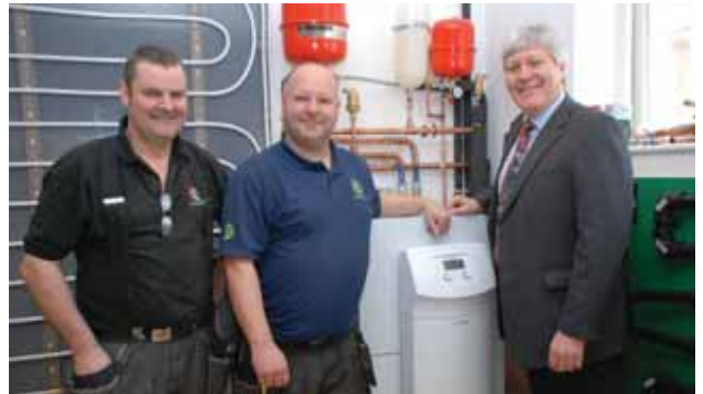
Team work: GroundTherm has recently carried out work at Manchester College, L-R Andy Major, technical advisor, Andy Louth and Bob Barlow, Star Centre
