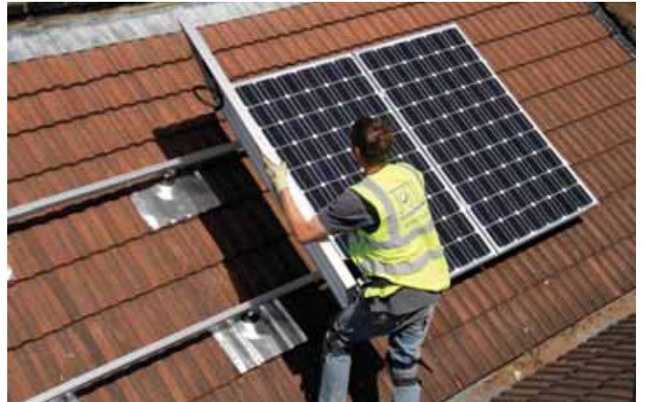
Money talks: Installers Joju Solar says the cost of installing PV systems at commercial premises is now cheaper and more cost-effective than it has ever been
