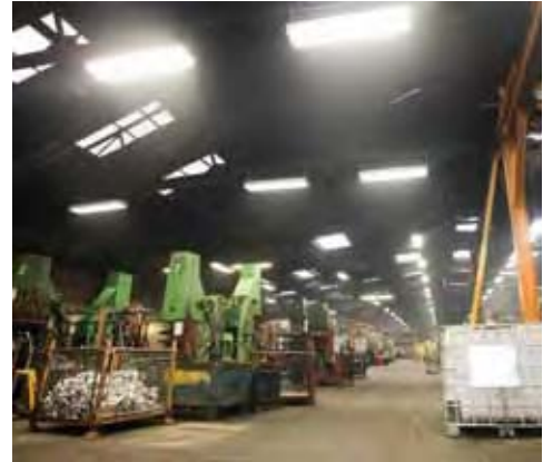
Bright idea: Lupton & Place foundry's £20,000 investment in energy efficient lighting should payback in just 2.5 years
