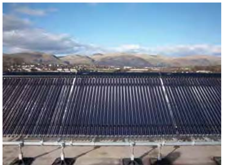
Hot property : Forth Valley College. Kingspan has installed 360 solar thermal vacuum tubes at two campuses
