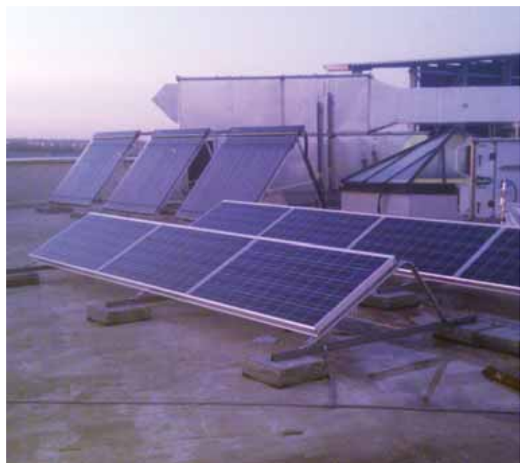
Green light: Doncaster's Flying Scotsman NHS health centre now boasts PV and solar thermal systems
