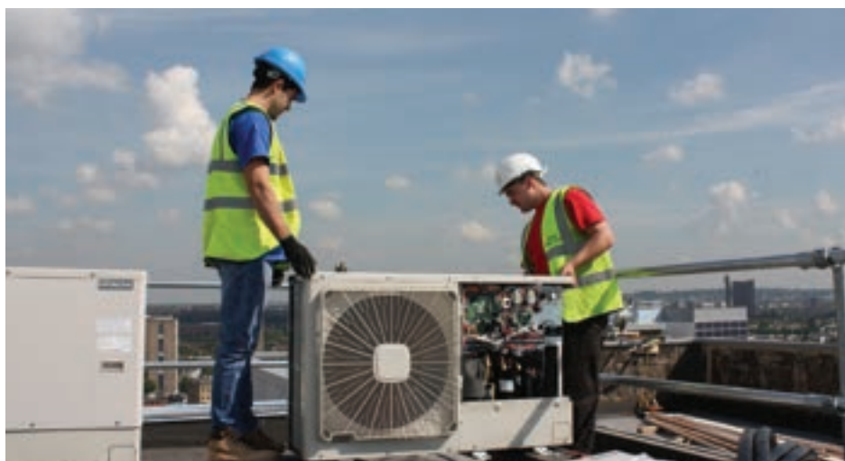
Premier event: Edward Woods Estate was the first project to incorporate Nu-Heat's new hot water cylinder, the Energymaster HP 255S
