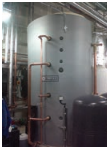
Smart technology: New for 2013 are Cordivari buffer tanks, available from Secon Solar
