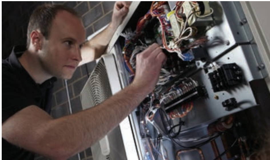
Perfect partners: According to Nu-Heat the relationship between installer and supplier is key to the success of a heat pump installation
