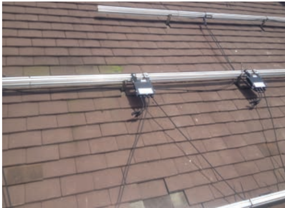
Laid bare: The power optimisers of the SolarEdge system, installed behind each panel, are designed to increase energy output from PV systems by constantly tracking the maximum power point of each module individually
