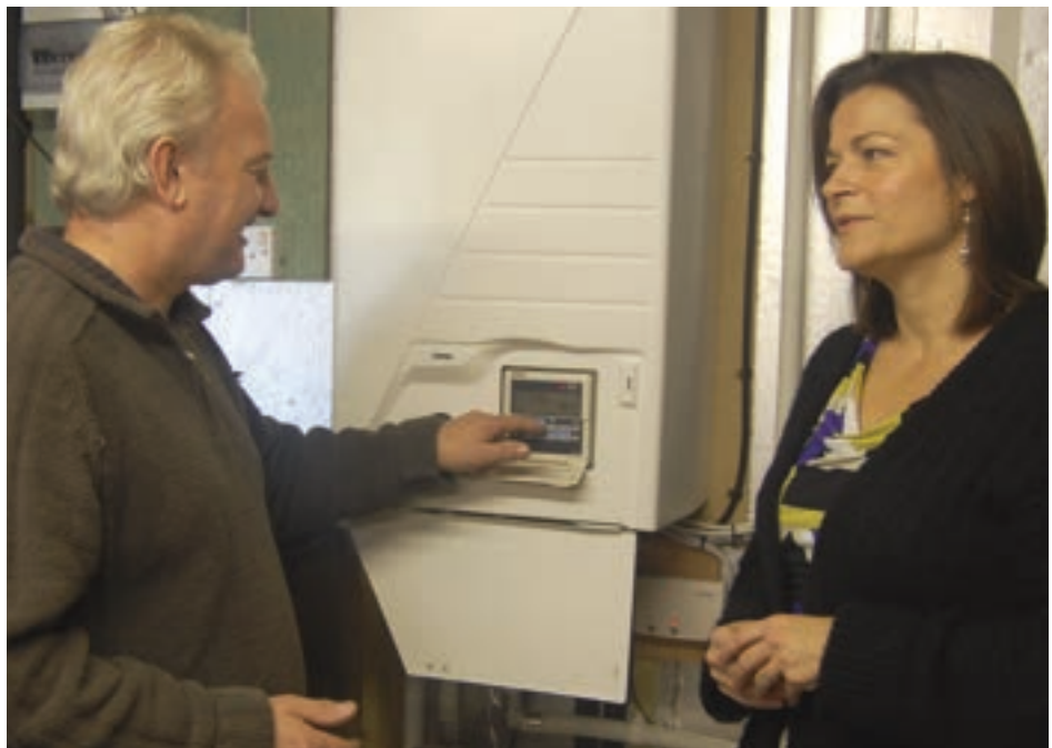
User friendly: Choosing a heat pump system with clear and simple controls is crucial if end users are to be comfortable adjusting settings
