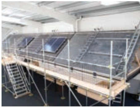
Real deal: The NAPIT Bristol Training Centre features fully functioning solar PV/thermal, combined heat and power pump and biomass installations
