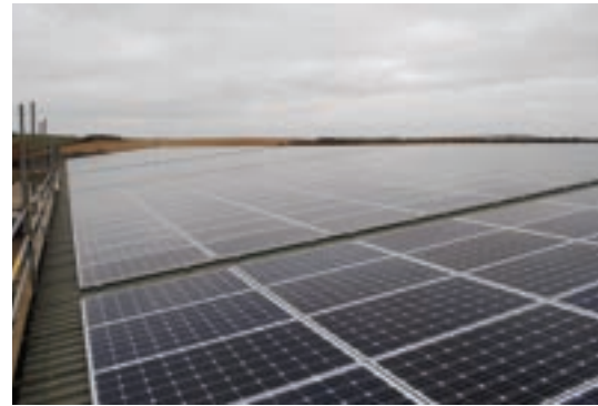
Go west: The Rand Brothers' 526kWp installation has been fitted on an east/west orientation to increase the hours of electricity generation
