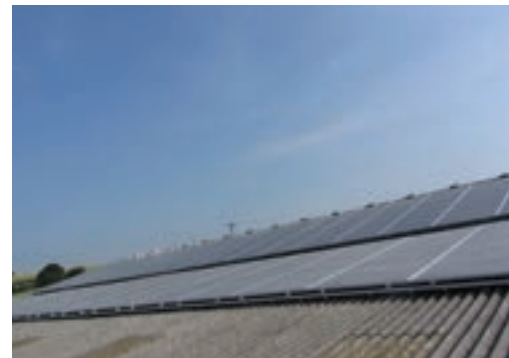
High society: Whitefield Farm owner Nigel Darwin predicts annual savings of £8,000 on electricity bills from his 50kW PV array
