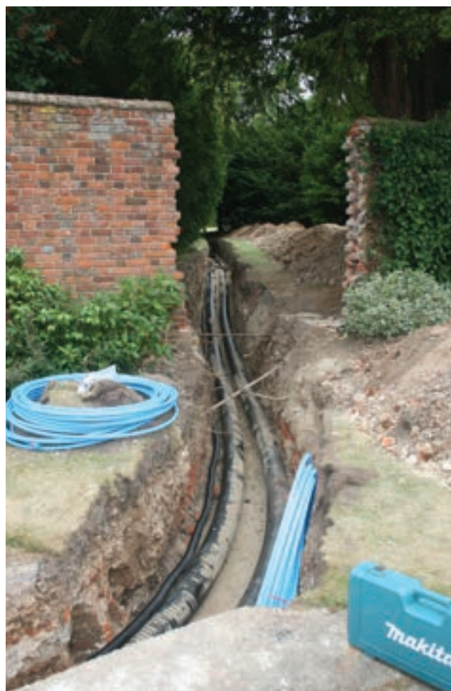
Going underground: With its sub-surface pipes, district heating can be an excellent way of supplying renewable heat whilst maintaining the historic and rural character of certain properties
