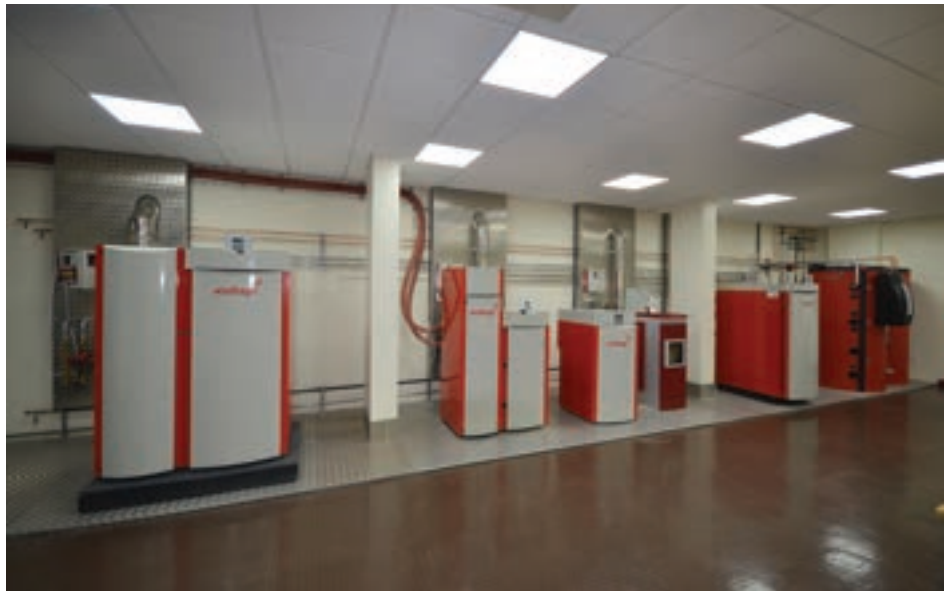
Well stocked: The training centre at Windhager is fully equipped with a full range of working wood pellet and split log boilers for effective training
