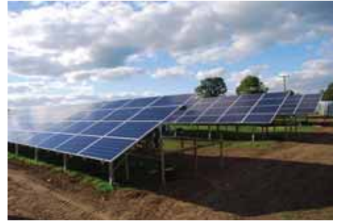
Power surge: Almost 4000 PV panels have been installed at Wedmore's new community-owned solar power plant, which is now feeding electricity into the grid
