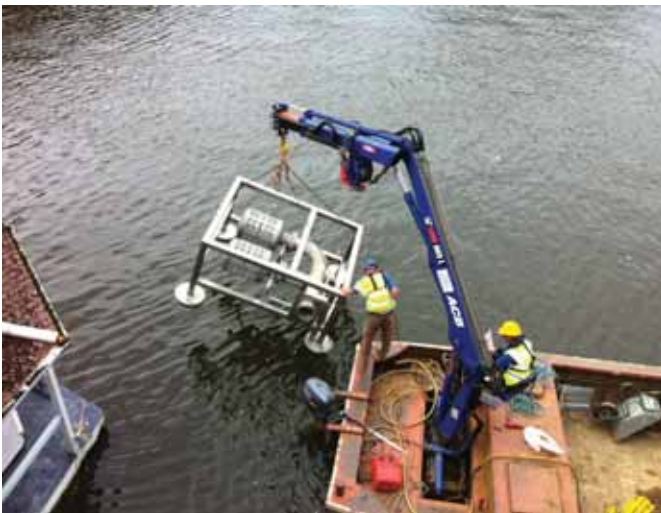
Liquid gold: Up to 13 million litres of water are drawn from the River Thames each day through high efficiency heat exchangers
