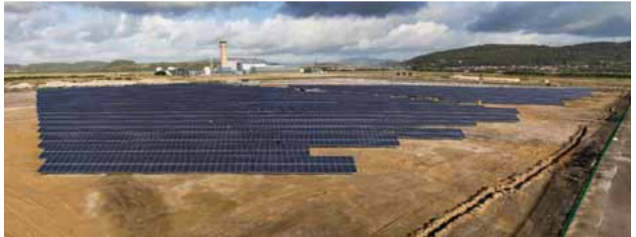
Urban decay: The 20,000 panel PV park at Baglan Bay, Port Talbot, is part of a larger £3bn regeneration project on derelict land in South Wales
