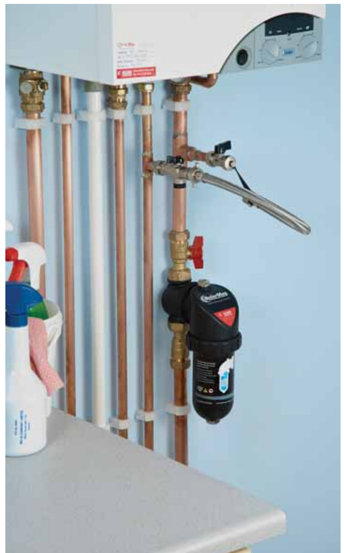
Heavy metal: As water circulates through the BoilerMag, ferrous sludge is removed via magnetic filtration, says the product's manufacturer Eclipse Magnetic
