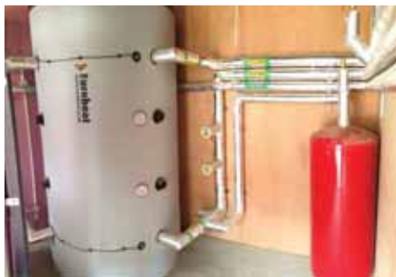
Healthy return: Eildon Cottages' new biomass system delivers combined fuel savings and an RHI income of £11,067
