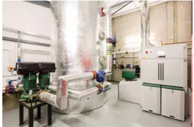
On the edge: The boiler house was built away from the main buildings to reduce the impact of wood chip deliveries
