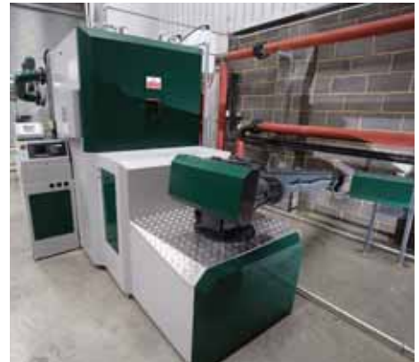
Above and beyond: Paul Clarke, Rural Energy, is calling for an MCS-equivalent accreditation scheme for biomass installations larger than 45kW
