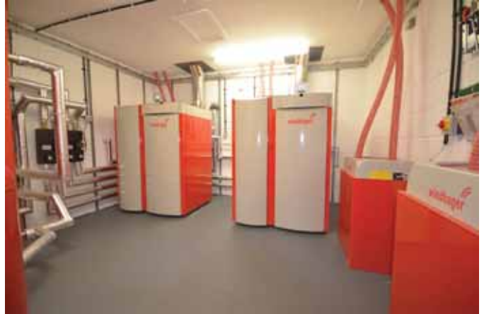
Old money: Two 60kW BioWIN wood pellet boilers from Windhager have netted The Manor House Golf Club substantial fuel savings on oil
