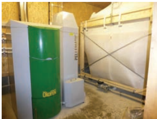
Golden era: Tropical Energy's ÖkoFEN Pellematic PES 56kW wood pellet boiler is netting the Welsh honey producer almost £30,000 a year through energy bill savings and RHI income
