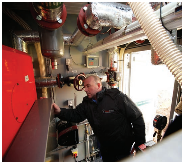
Words of wisdom: Tim McLeman of Wood Energy warns that as RHI payments are tied to a product by its serial number, it is vital these technologies last for the full 20 year term or all future payments are lost, underlining the importance of an effective warranty
