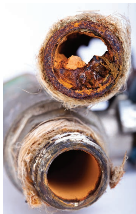
Down the tube: Choosing the right heat transfer fluid can have enormous financial implications for heat pump systems despite its low capital outlay, says Kilfrost
