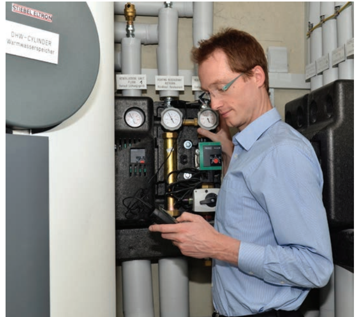
Fine tuning: Educating consumers on the advanced settings of heat pumps and customising systems for their individual needs can provide installers with an added value service, says John Felgate, Stiebel Eltron
