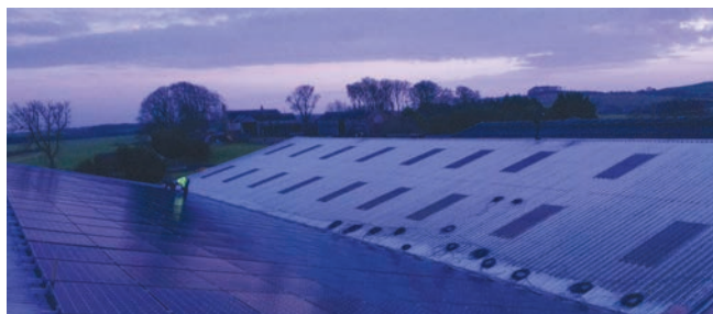
One and only: The 150kW, 460 panel PV system at Hulam Farm, Durham is understood to be the largest privately owned system in the North
