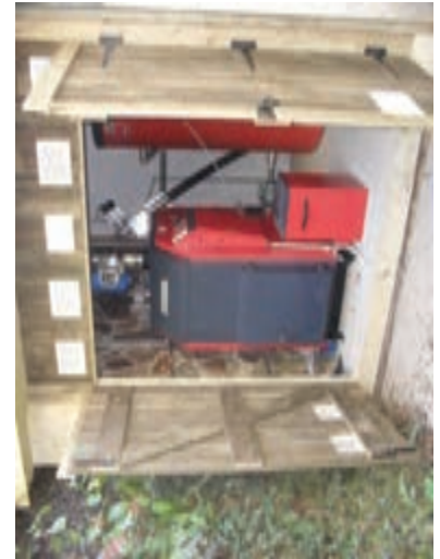
Hot stuff: A Strebel Taurus ST75 boiler sited in a converted garage now heats Heddons Gate Hotel in Exmoor
