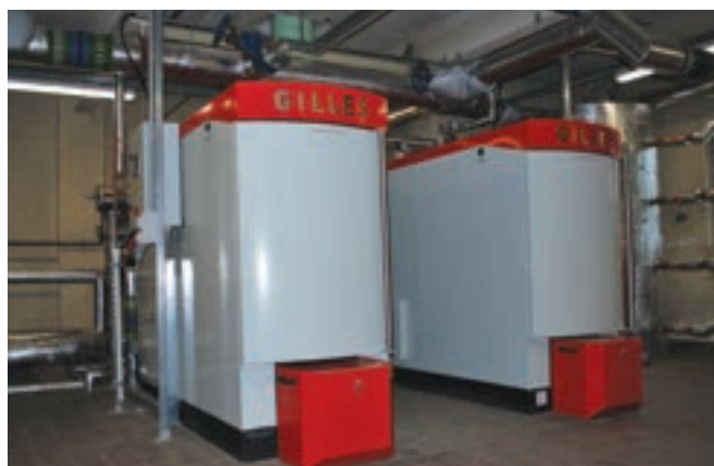
Air strike: The RAF has slashed its annual emissions by over 300 tonnes having installed 775kW of biomass capacity at its largest base Brize Norton
