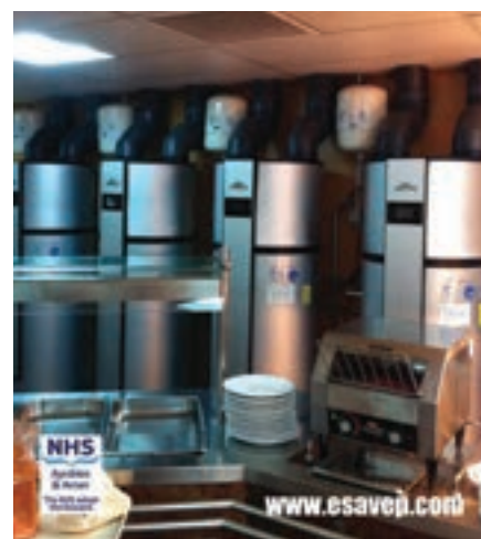
Fan club: Ecocent heat recovery and ASHP units have not only reduced the cost of producing hot water at Crosshouse Hospital, Kilmarnock, but also negate the use of expensive extractor fans in the kitchen areas
