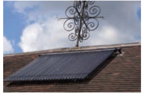
Liquid gold: Solar thermal will contribute towards a 32 percent bill saving alongside biomass at a Solihull stable conversion, having replaced an old oil-fired boiler
