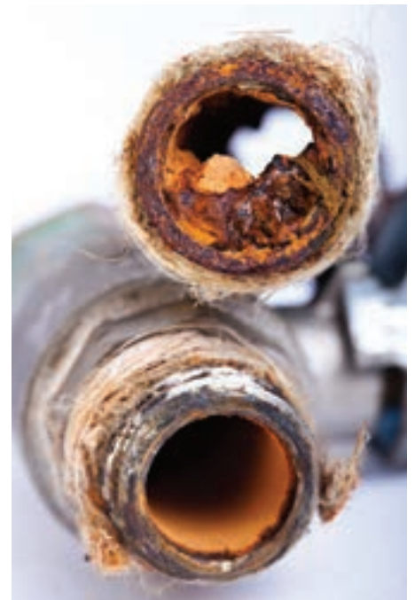
Long game: Using high quality heat transfer fluid is a simple way to achieve long term savings in heat pump systems via corrosion reduction, says Andrew Murray, Kilfrost
