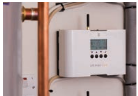
Numbers game: 4Eco's immerSUN has helped over 17,000 UK homes to reduce their energy bills and increase self consumption of renewable energy
