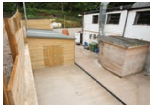
Smart money: Glan yr Afon Inn can now add £9,000 to its annual income from its 80kW wood chip boiler under the RHI
