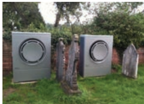
Heaven sent: Shirley Parish Church, Derbyshire, is now a more comfortable space for worshipers after replacing ineffective electric tube heaters with the power of air source heat pumps
