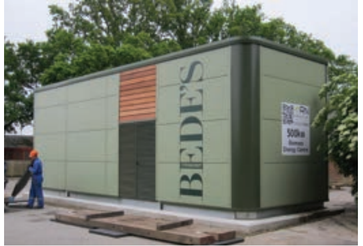
Money box: A £1.2m investment in biomass by Bede's School in East Sussex was facilitated by Siemens and the Carbon Trust's Energy Efficiency Financing Scheme (EEF)
