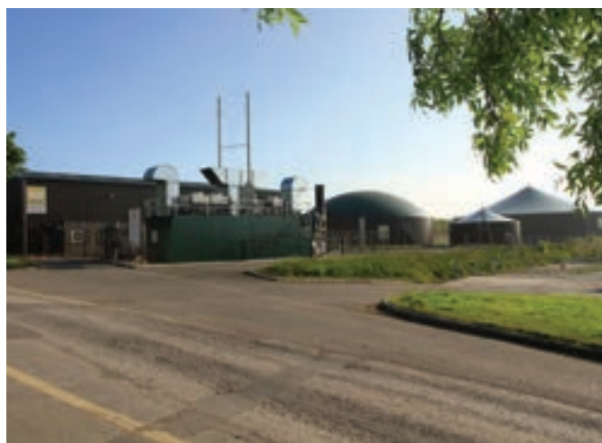
Smell of success: After two years successful operation, Weltec have been chosen to build a 1.1MW extension to the Piddlehinton food waste AD plant
