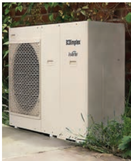
Above: An air source heat pump
