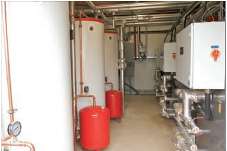
Top: The heating system at RAGT Seeds and below, the company's plant room
