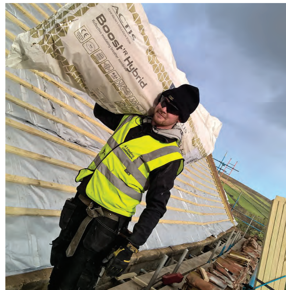
Above: Preparing the roof of Danby Castle with the Actis Hybrid insulation system.
