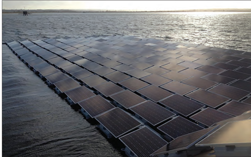
Above: Europe's biggest ever floating solar panel array on London's Queen Elizabeth II reservoir as part of Thames Water's ambitious bid to self-generate a third of its own energy by 2020.
