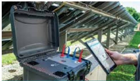
Taking measurements using the Sonel MZC-340-PV meter
